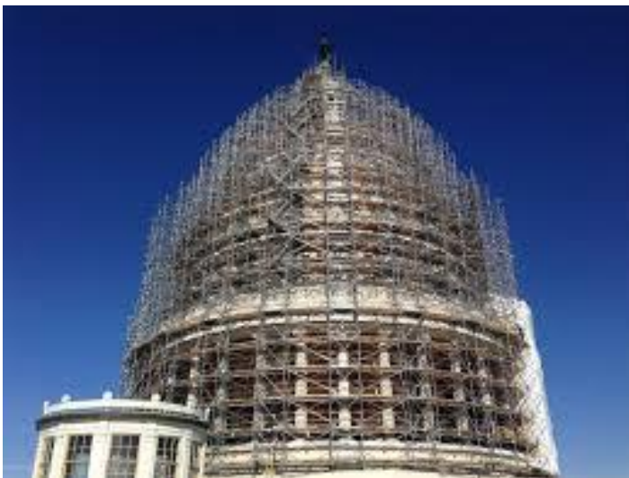
The Capital Dome with surrounding scaffolding for repair of damaged and structural weakness is analogous in appearance and inherent weakness to the original tower of Babel in the Bible. Departing from God, any nation will fall, along with its proud monuments. (Isaiah 9:9-11; Revelation 18:9-10)
